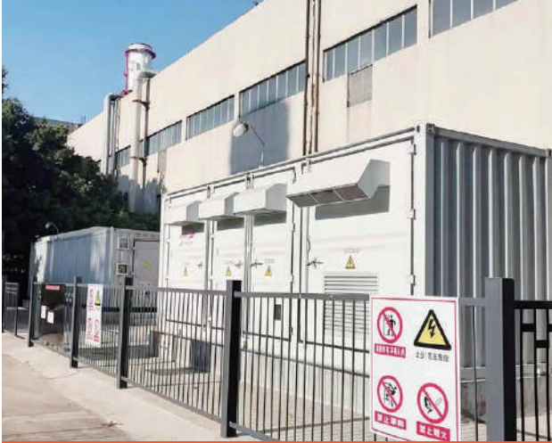
◎ Shenzhen Nanshan Power Plant Frequency Modulation Project
