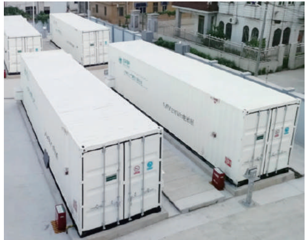
◎ State Grid Zhenjiang Changwang Energy Storage Project
