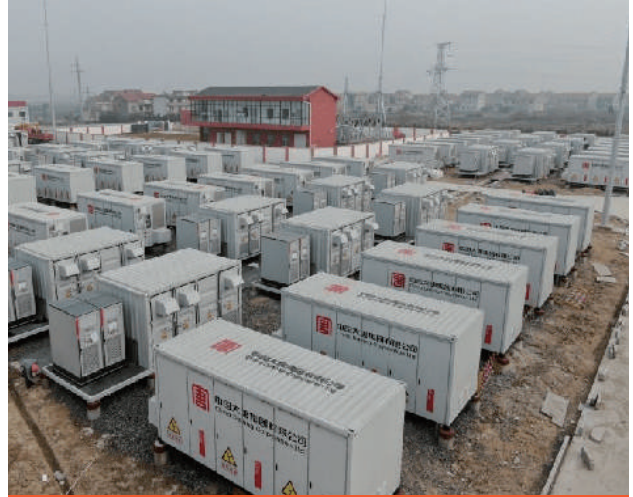
◎ Datang Longgan Lake Energy Storage Power Station Project
