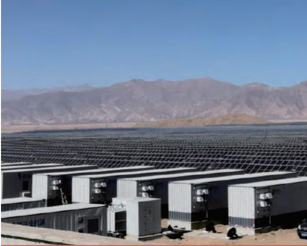
◎ Tibet Light Storage Comprehensive Energy Project
