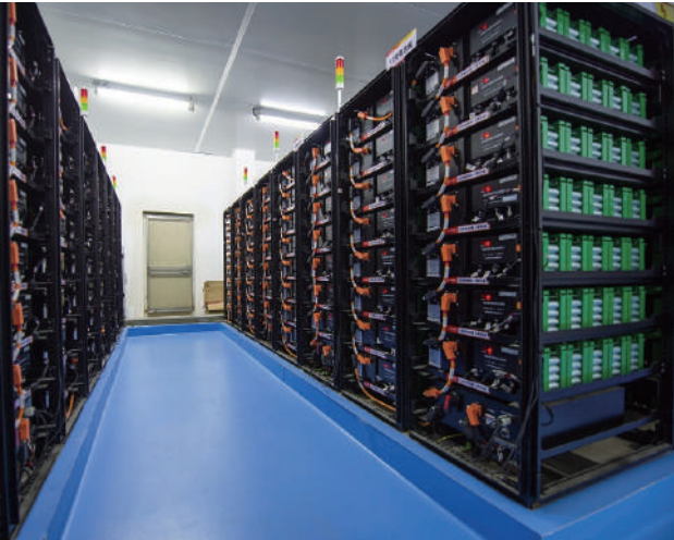
◎ Kunshan Industrial Park Energy Storage Project
