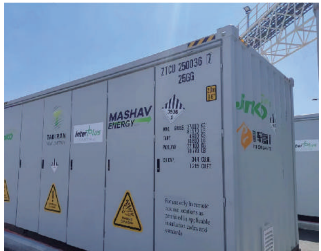
Europe Storage Project
