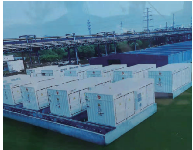
◎ Zhangjiagang Yonglian Steel Plant Energy Storage Power Station Project
